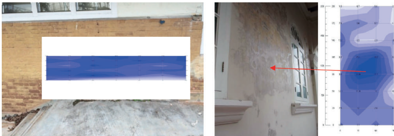
Figure 3. The tomograph on the left indicates rising damp on a masonry wall. Localised spot of dampness could be picked up within a wall as seen in the right tomograph with the damp wall shown in the centre.
